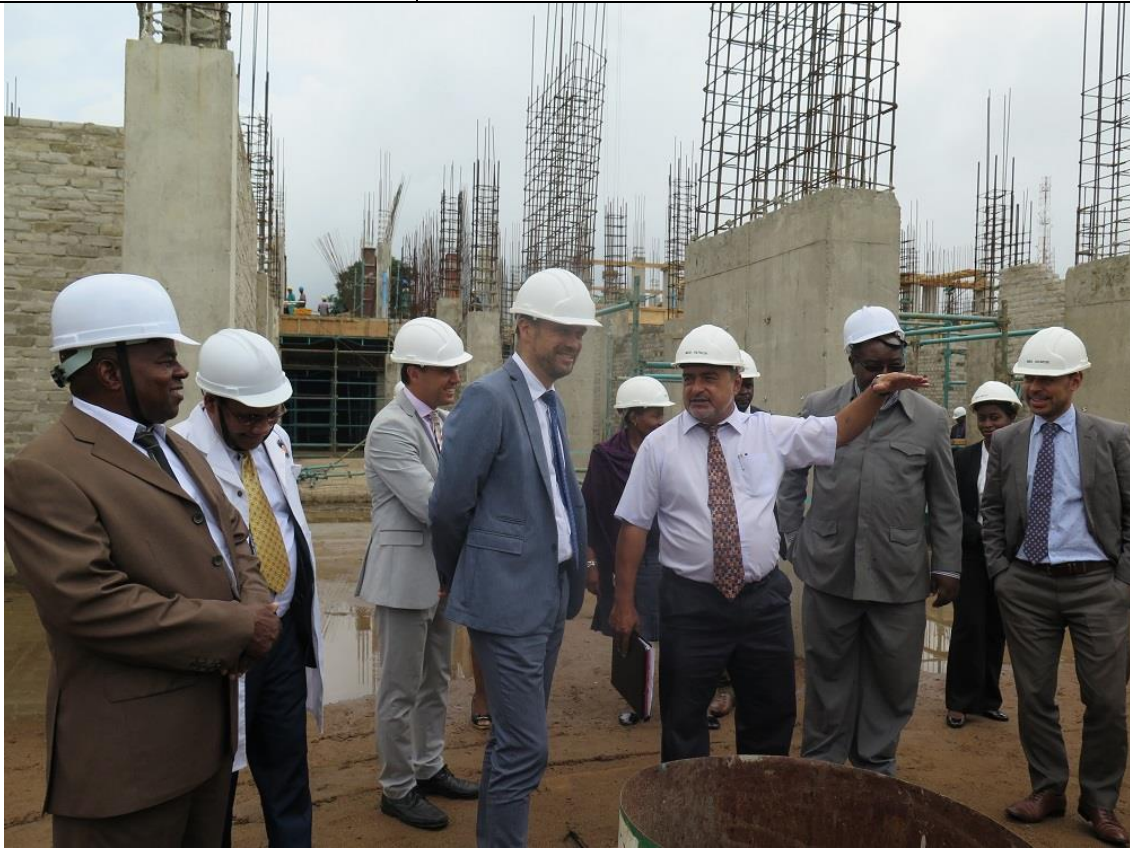
Photo taken during visit of the EU Delegation to the new MBS Laboratory Complex Construction Site
